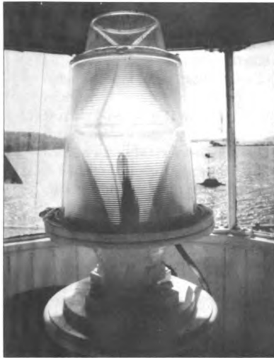
This solar-powered beacon was installed in the lantern in 1990. Photo by author. The beautiful sketch of Saugerties Light was done by Paul Bradley Jr.
